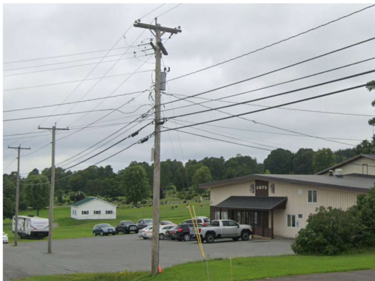
Figure 11 24 Houlton Road Electrical Connection
